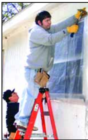
KEETOOWAH CHEROKEE CASINO maintenance employee, Dustin Sanders, right, and Hominy Littledave, left, UKB Community Service Coordinator, volunteer their time to help repair and winterize a Keetoowah Cherokee elder's home.
